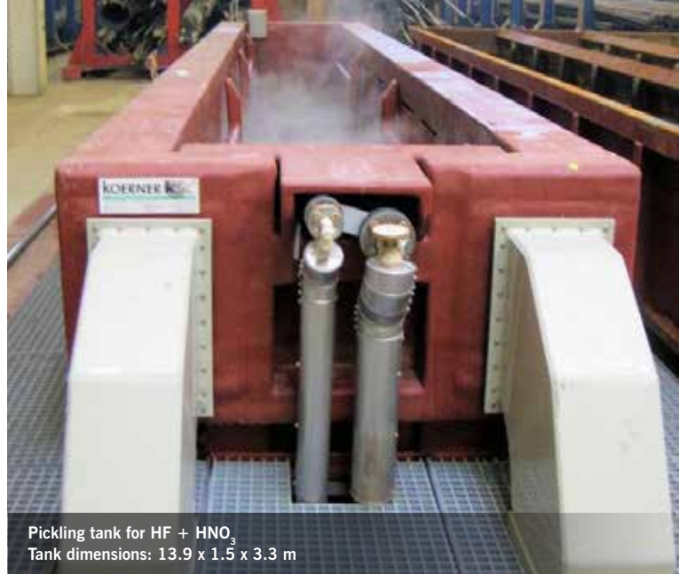
Encapsulated tube pickling plant Tank dimensions: 11.0 x 1.2 x 1.65 m
